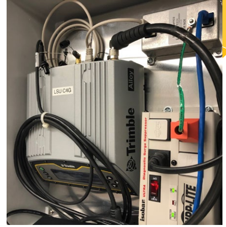
Inside an LSU C4G GNSS base station enclosure that has access to Ethernet and AC power.
